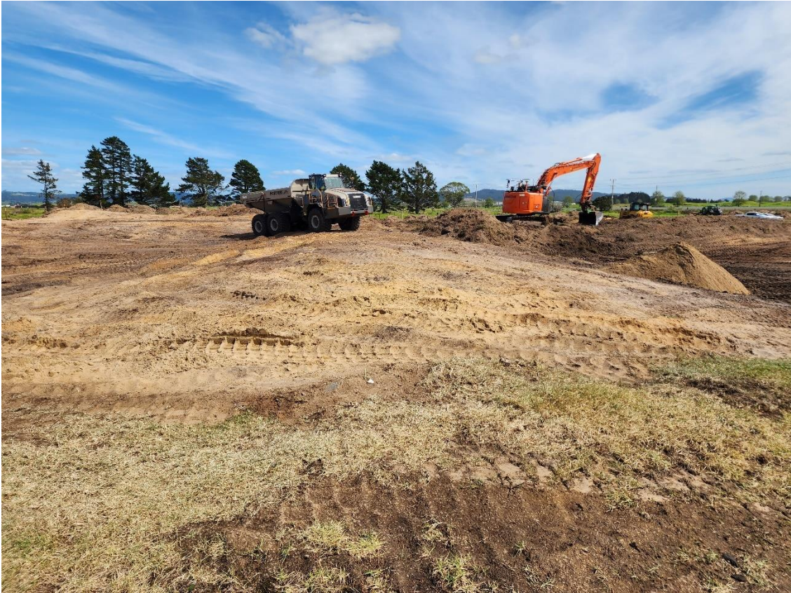
Figure 40: Looking west over the BESS site while monitoring on Site 1 (2023).
