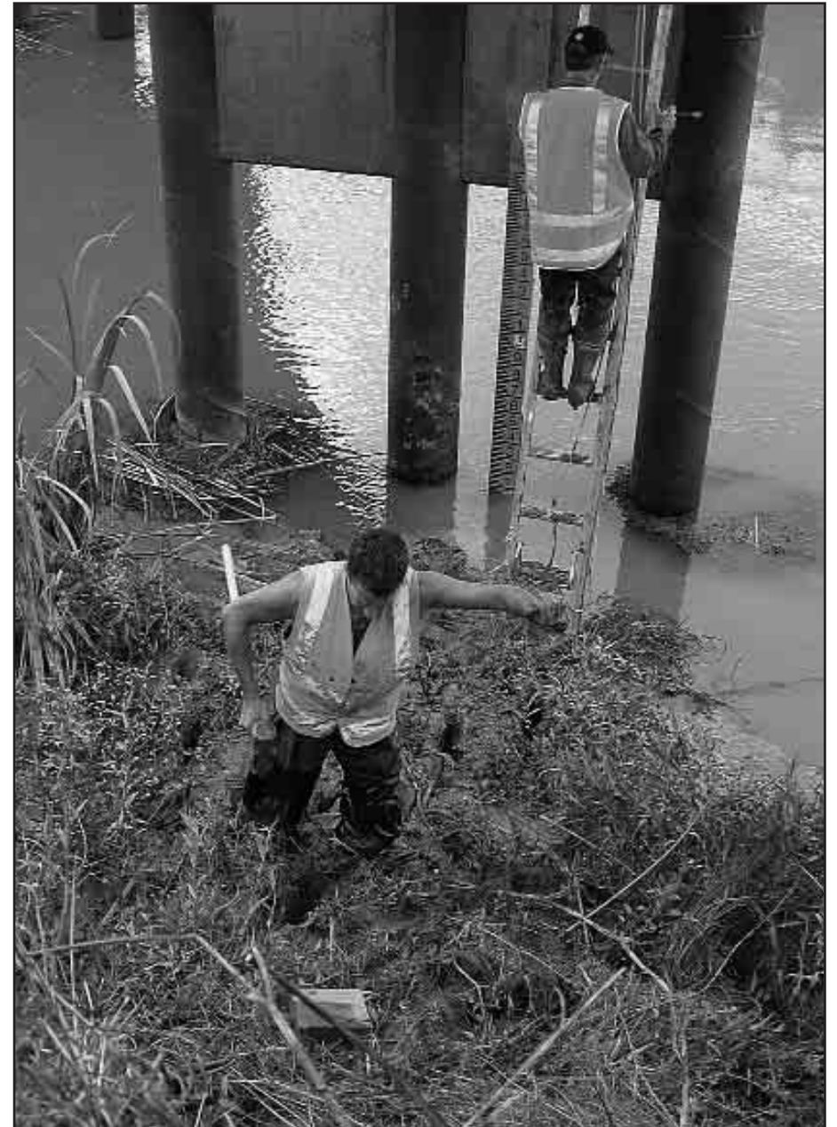
Regional Council Hydrology staff install a new water recorder on the Lower Kaihu River.
