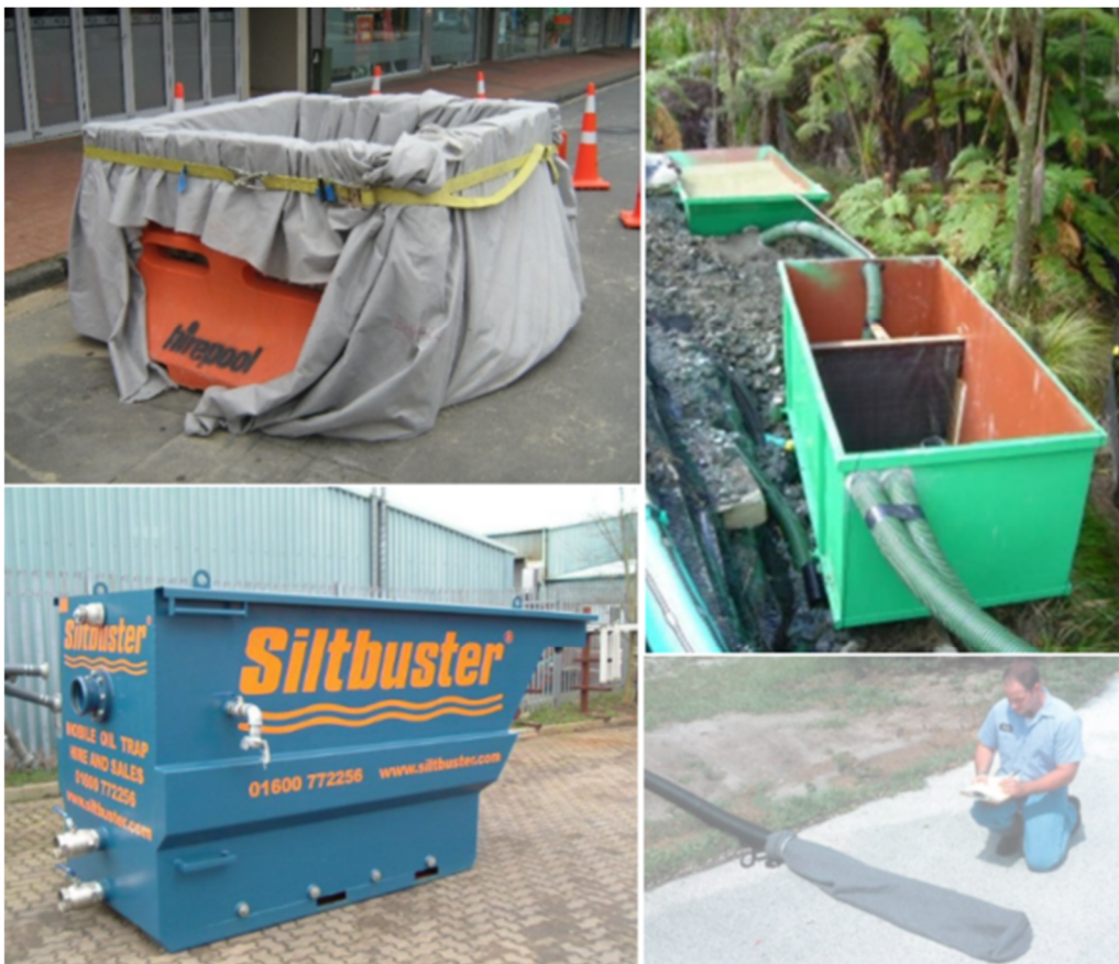
Figure 6: Example dewatering devices, clockwise from top left: turkey's nest, baffled skip bins, small dewatering bag, lamella clarifier.
