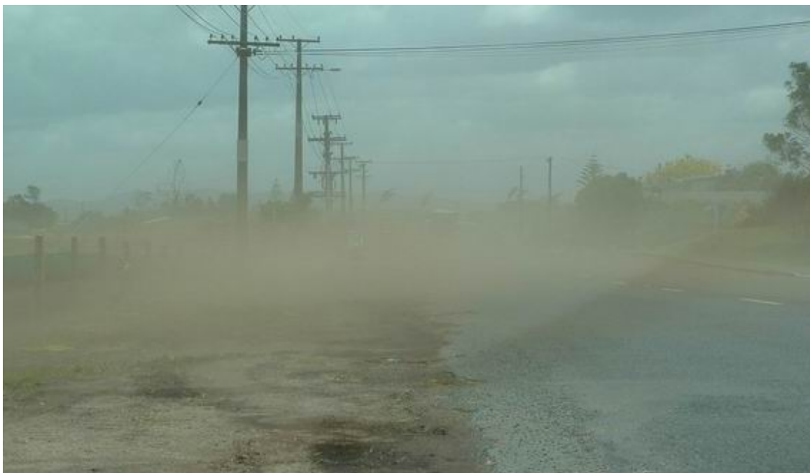
Dust originating from the earthworks (on left of photograph) being blown across the road towards residential properties on the right.
