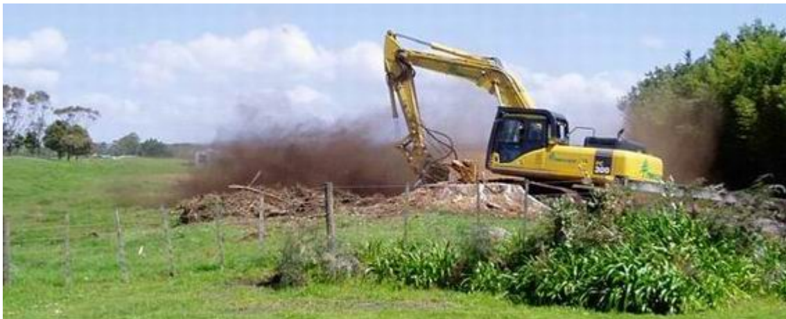
Digger generating dust, while excavating trees in the One Tree Point area.
