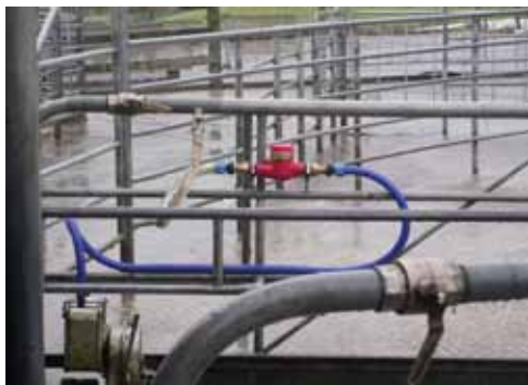
Water meter on backing gate at Mayflower farms.
