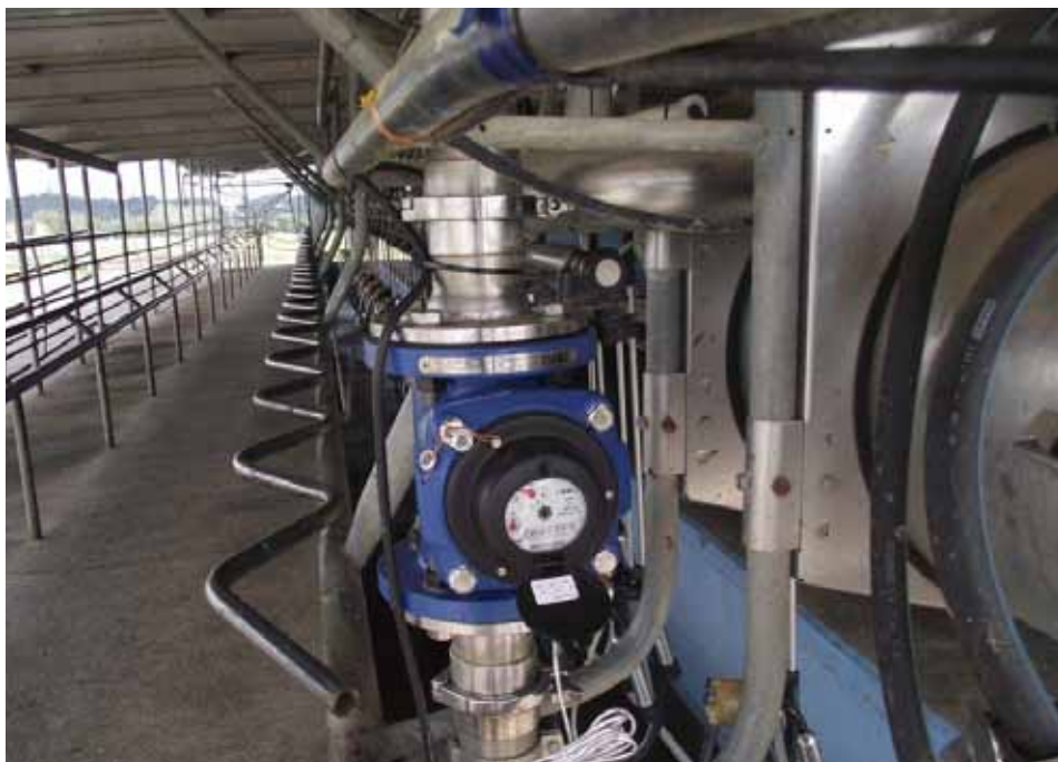
Multiple meters were installed during the trials on both farms.
