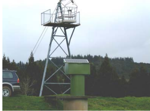
Water Level Telemetered Station – Whakapara River at Cableway
