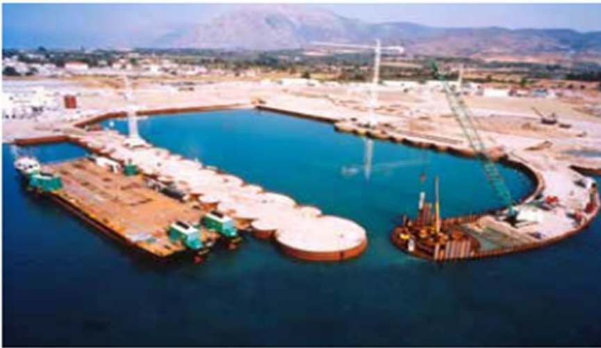
Figure 41: Concept interlocking circular caissons with gravel or sand infill (WSP Concept Design Report, 2022)
