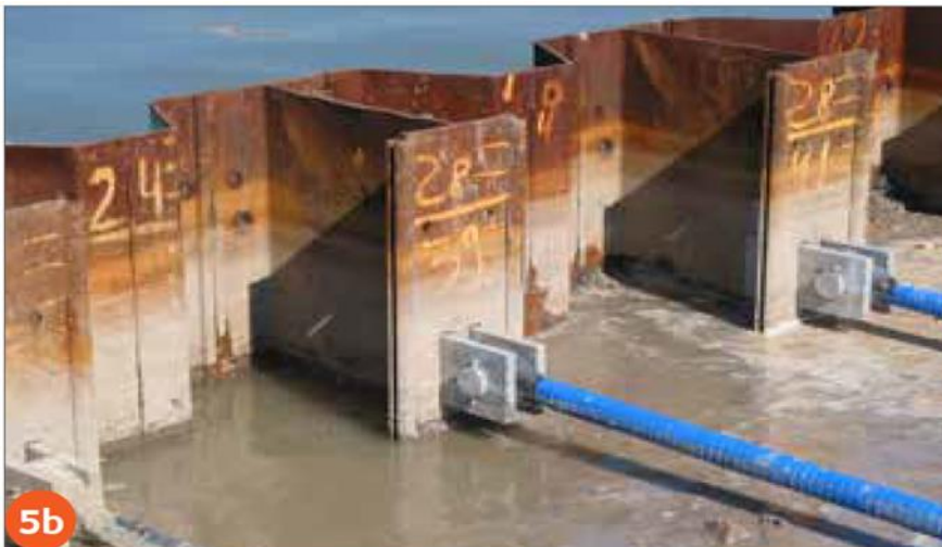
Figure 42: Concept single combi-pile wall with tie back anchors (WSP Concept Design Report, 2022)
