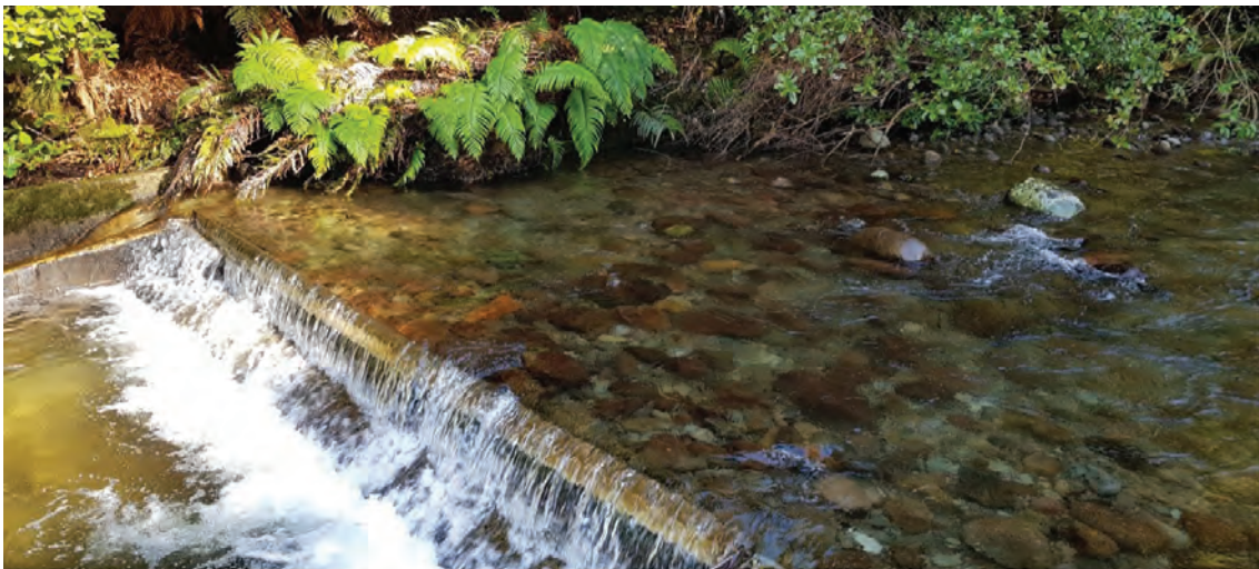
A weir at Manguika Gorge, Waikato, used as an example during the NIWA Fish Passage Masterclass in May 2023. The vertical face would only allow a few native fish to climb up, but the metal lip at the top of the concrete face would make them slip back down. Upstream is amazing habitat for native fish but sadly very few can reach it.
