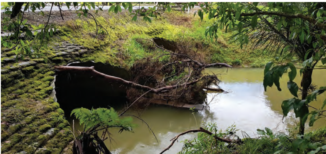
Example of a good double culvert system underneath Otaika Valley Road that would easily allow for fish passage and hasn't undermined the structure of the stream bank or altered water flows.
