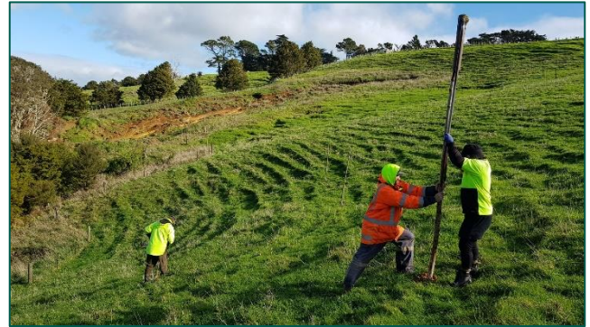
Contractors planting poplar poles to prevent slips like the one in the top left of the image.
