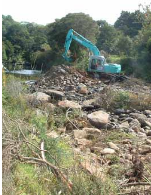
Kerikeri River, one of several locations at which minor river works were undertaken
