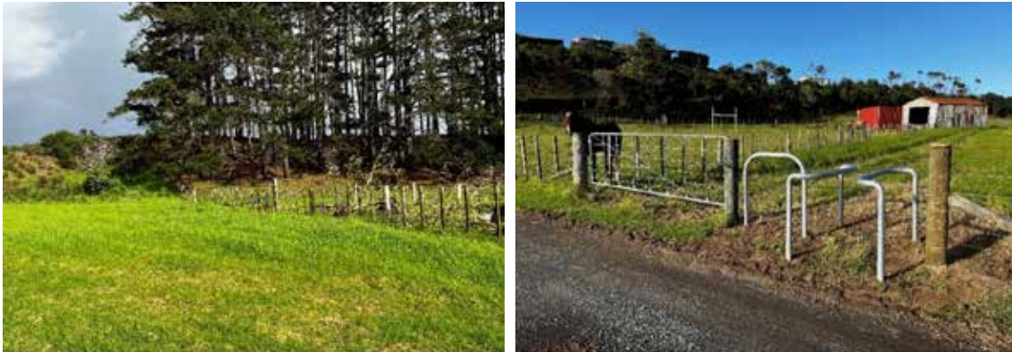
An old fence was repaired, and a new mountain bike gate installed at Lake Gem by Summit Forestry with support from the FIF Dune Lakes project.
