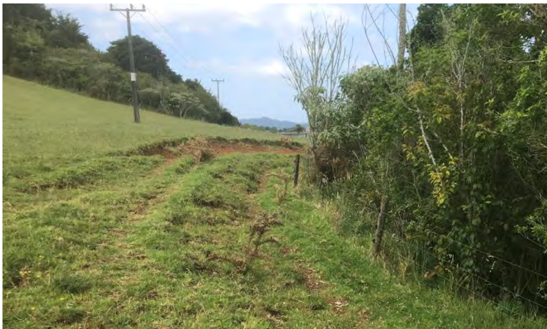
Figure 6: View east over the crest of the arcuate stream bank slope, showing area of erosion or livestock tracking.
