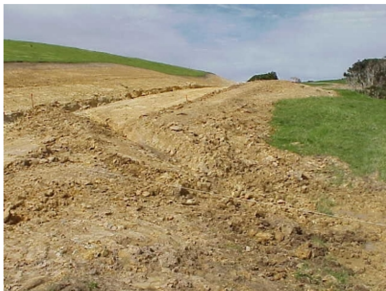
Photo: Earthworks on a slope without sediment control
