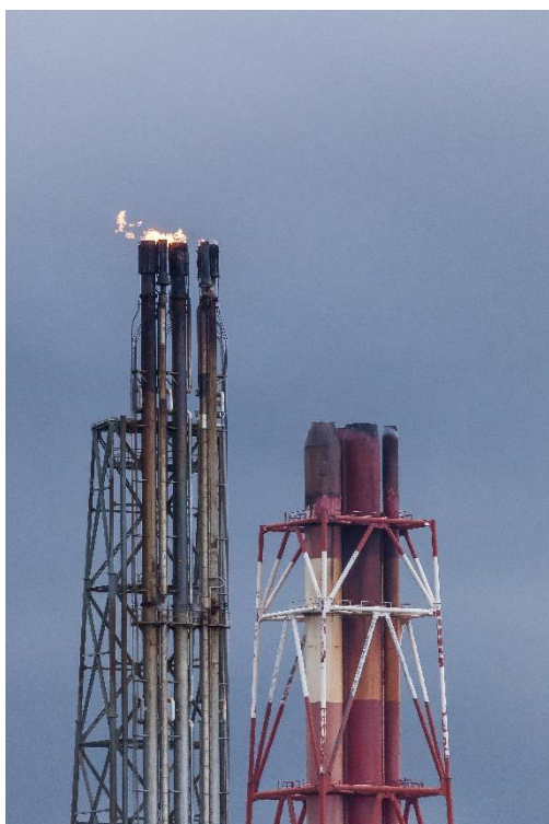
Figure 2.5: Photo of flares with the Block B, C and Utilities stacks in the background.
