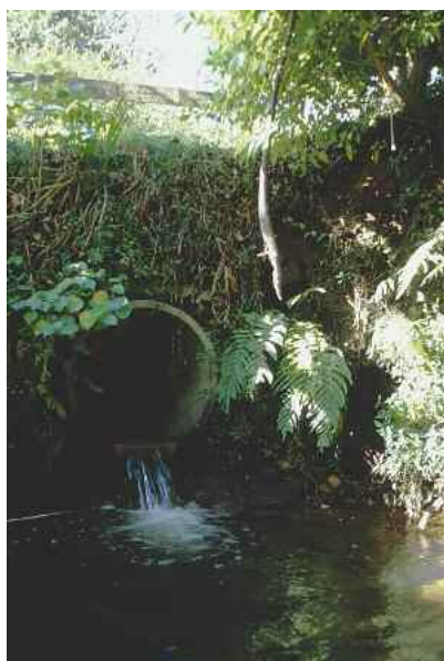
Poorly-designed culvert that is positioned too high in the streambed.
