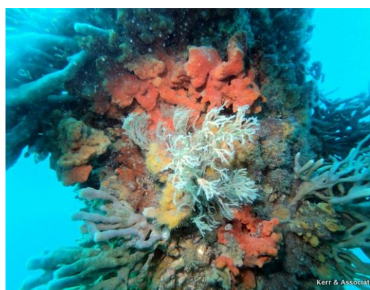
Photograph 2.3.5.6.2: Diverse encrusting assemblages on the Refining NZ jetty piles
