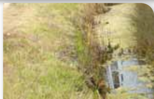
Algal growth in a roadside drain
