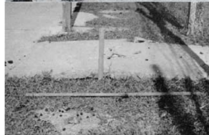
Otangaroa School. General view, and details of damage to concrete path. The rule lying on the grass in the lowest view is 1m long.
