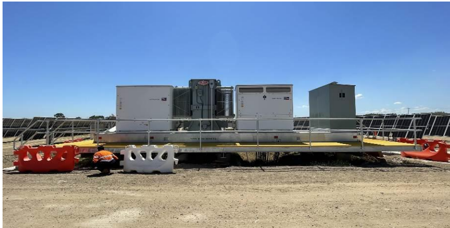
Photograph 12: An example of a typical inverter power station assembly. This is set closer to the ground than those proposed for the Ruakākā installations. Image source: Meridian
