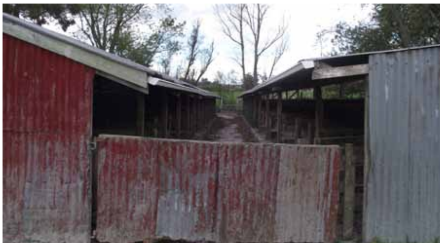
Guttering fitted to wintering barns to reduce effluent volumes
