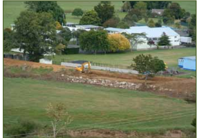
Work to rebuild the Kaeo stopbank is one of a number of flood risk management strategies completed in the past year.
