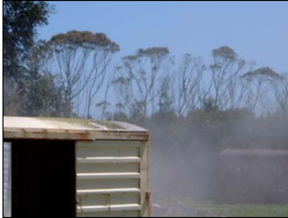
Dust nuisance caused by abrasive blasting
