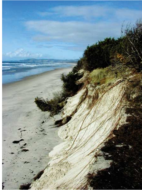
Figure C.2: Erosion scarp along the Pakiri-Mangawhai coastline in 2001 at the end of a La Niña period. [Photo: RK Smith].
