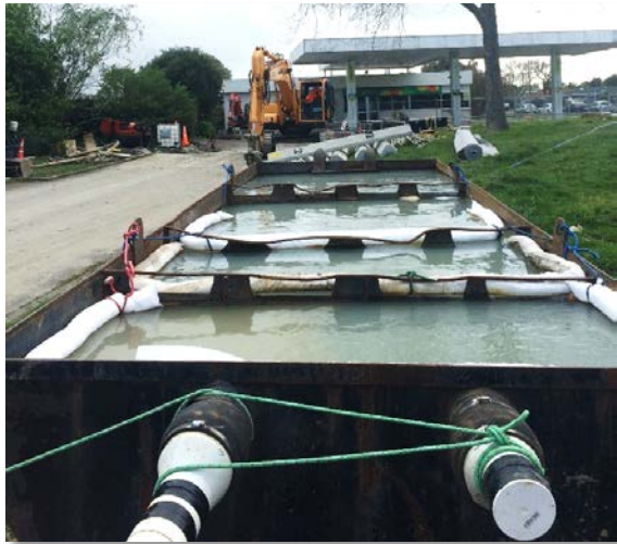
Photo 2: Settling tank with baffles and booms
